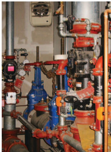
A recently completed fire protection system project.
